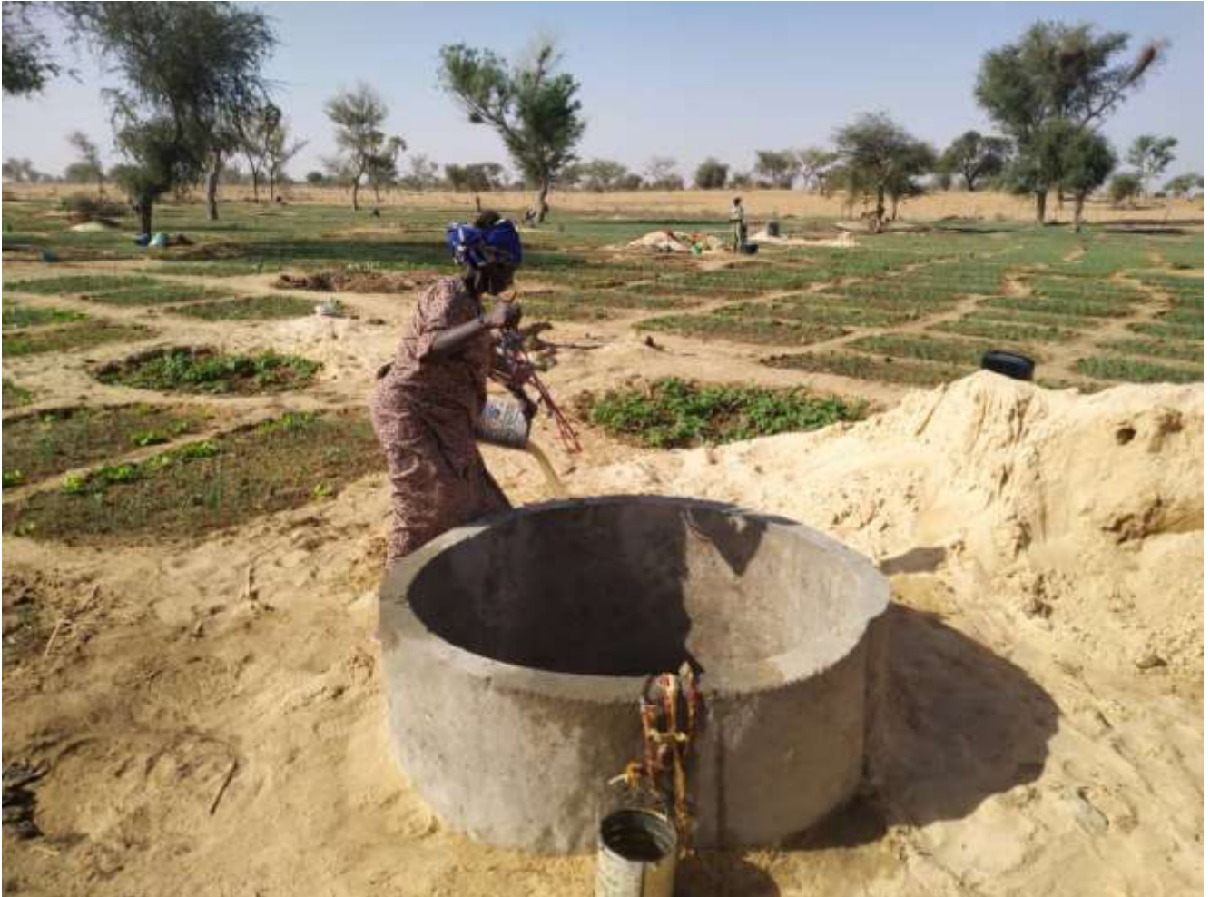
The new well of Ouddé Seybou in the rural commune of N'gonga
